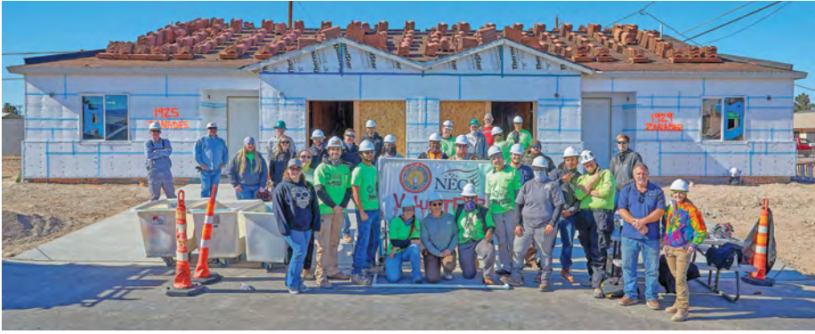
Local 357 members volunteer for the Habitat for Humanity Pittman Project in Henderson, NV. Photo courtesy of Carole Kilburn.
